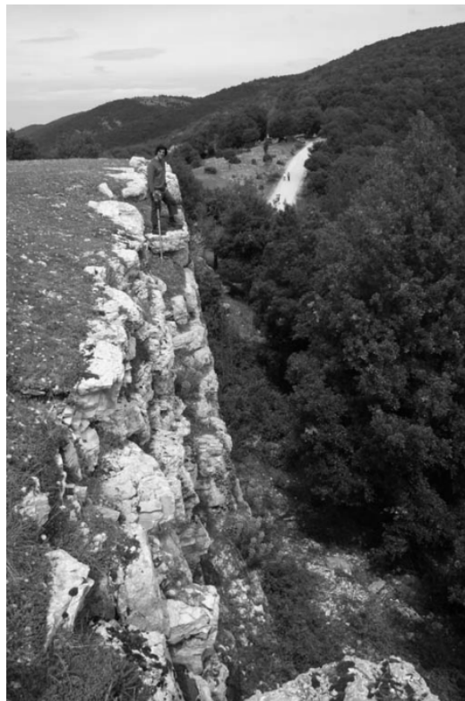
Fig. 6. Author Nicola Schiavottiello surveying the steep north-east corner of the building, looking north to the Martani mountains
