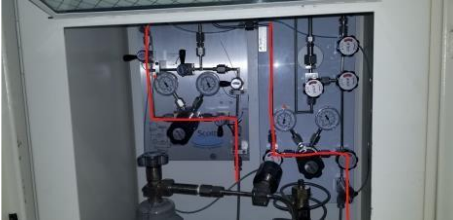
1 - Image illustrates the Cl 2 and BCl 3 gas lines near cylinders. CW turns to close the cylinder.
