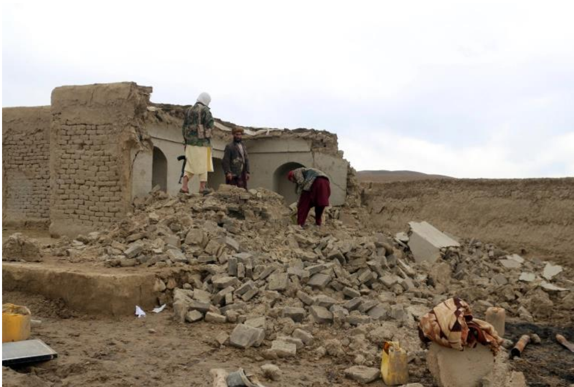
Damage to an adobe structure in Badghis, January 2022. Taliban soldier guarding the location.
