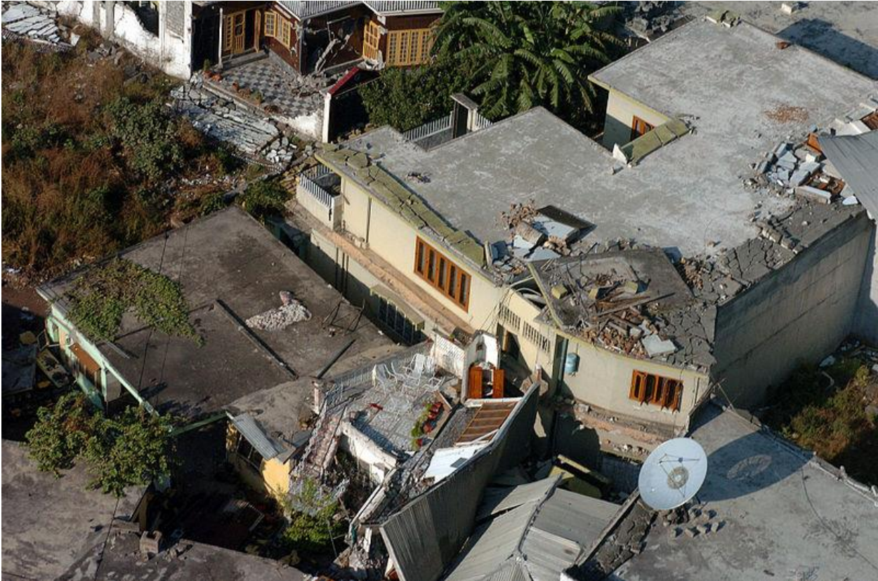
Damage to an RC building in the northwestern towns of Pakistan due to the 7.5 magnitude earthquake of 2015 centered in the Hindukush region.
