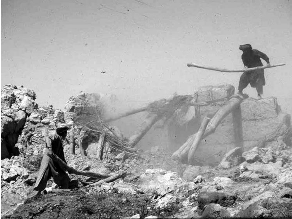
After a damaging earthquake, these villagers are digging into the debris to save a few wood planks that might have not been damaged. These wood beams are used in roof structures.
