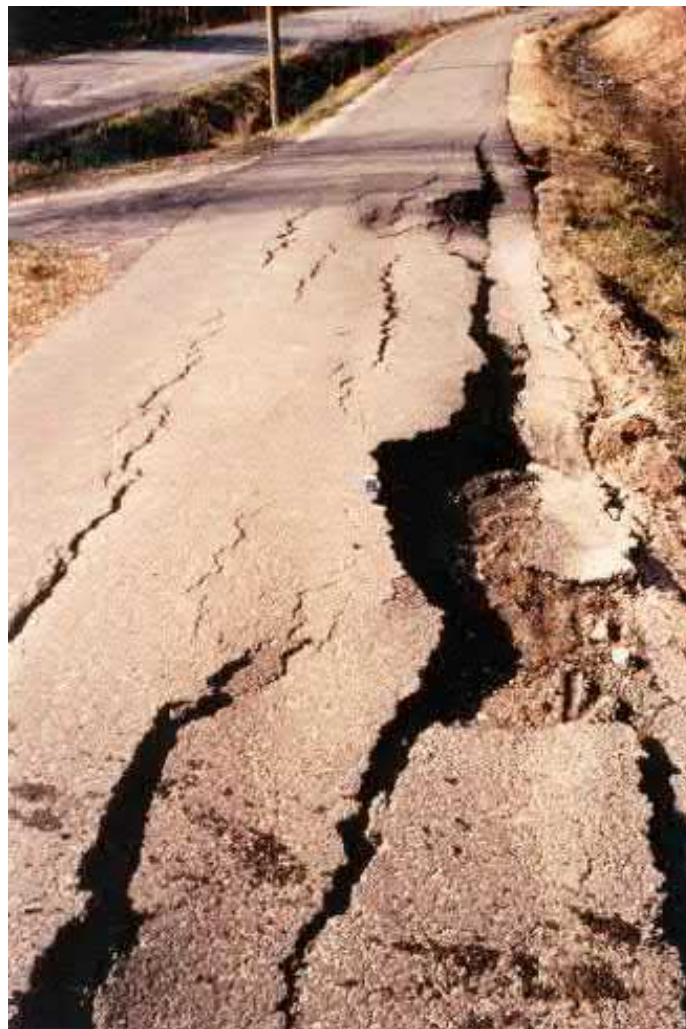
Figure 7.18: Damage due to frost heave near Jyväskylä, Central Finland in 1981. Photo: Risto Virpimaa (Photo collection of the Finnish Transport Agency/Mobilia museum, Kangasala).
