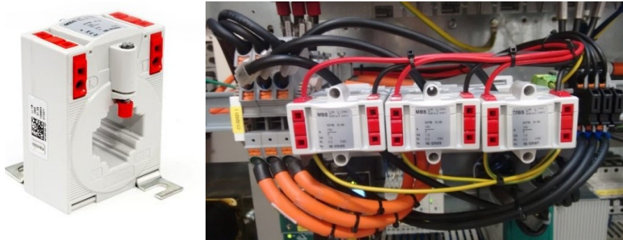
Figure 18 – MBS XCTB 31.35 transformer and its installation on the machine.
