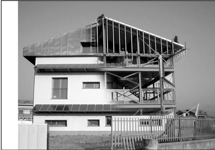
Figure 1: the South front of the house: left, in its final appearance; right, during construction.
