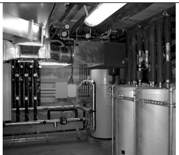
Figure 6: the technological installations at the underground level: above, the ventilation unit with heat recovery from exhaust air.
