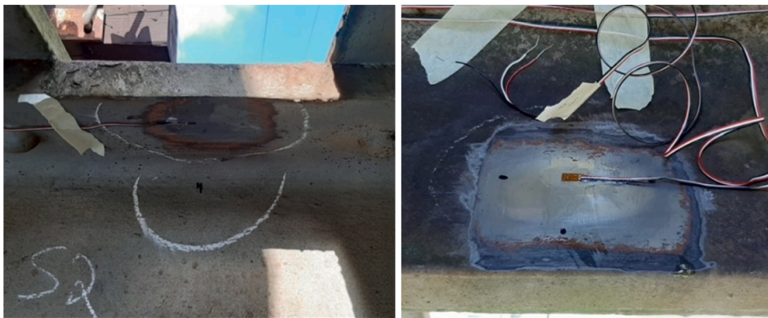
a) S2 (before the mechanical protection)
