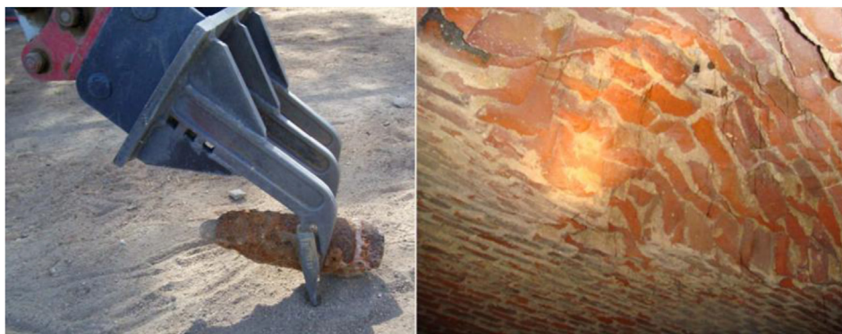
Figure 8. Shell found in the excavation during the operation and the detachment caused in the vault.
