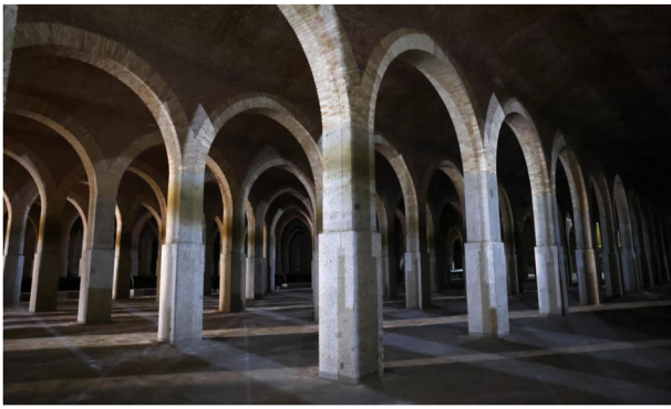
Figure 6. Interior view of the empty second (or Mayor) underground tank during the waterproofing works. Source: https://www.comunidad.madrid/ (Madrid, 2021).
