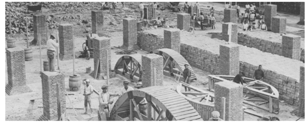
Figure 2. Construction of the Valencia water tank (1849–50) Source: Valencia History Museum, https://mhv.valencia.es (MHV, 2022).
