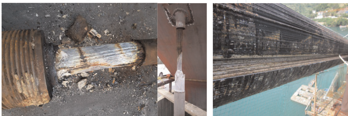
Figure 1. Corrosion and fatigue damage of cable-stayed bridges in mountainous areas with cable-stayed cable, suspension cable, and main cable.
