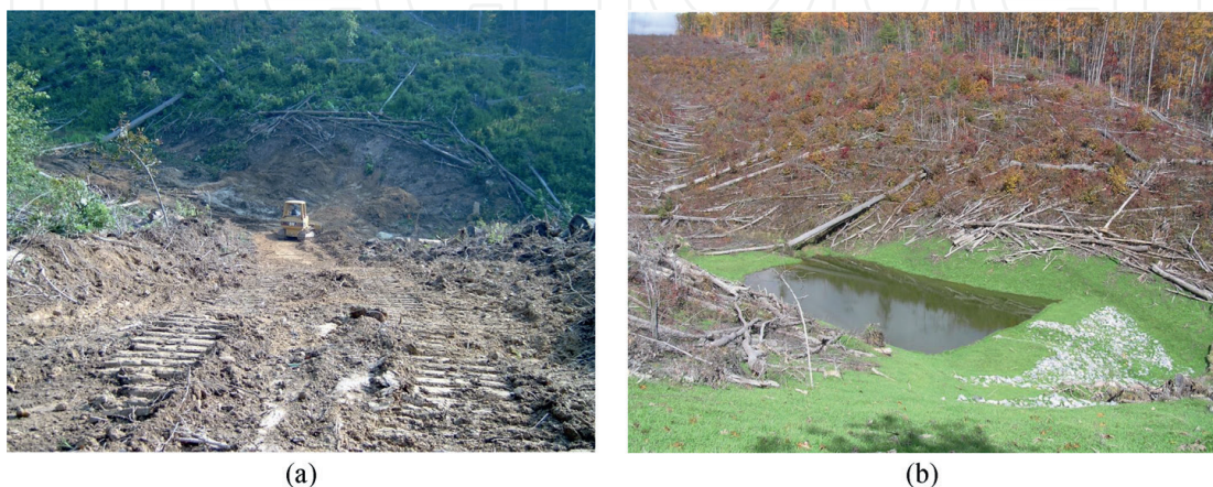
Figure 2. Pond site 22 construction (a) within and coincident with ROW development in August 2006, and (b) this same pond after first filling October 2006.
