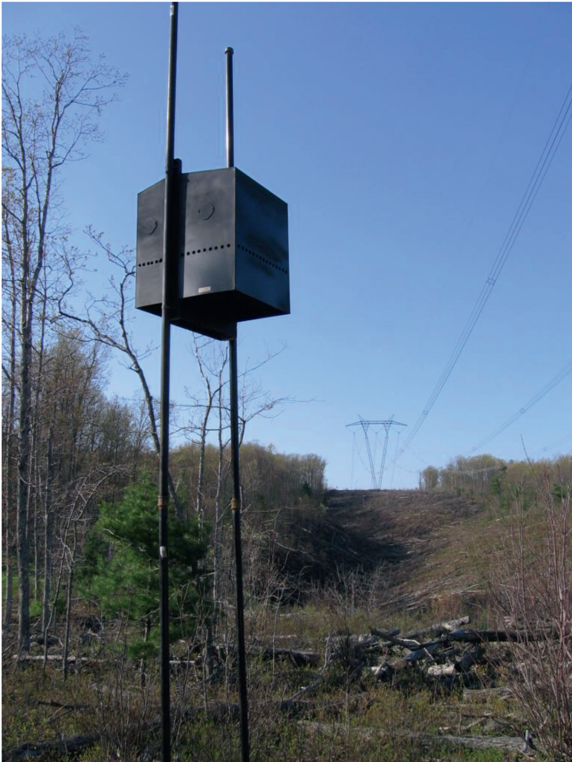
Figure 3. Small and large (7 and 24 chamber) metal-clad bat boxes erected on metal poles within the transmission line ROW.
