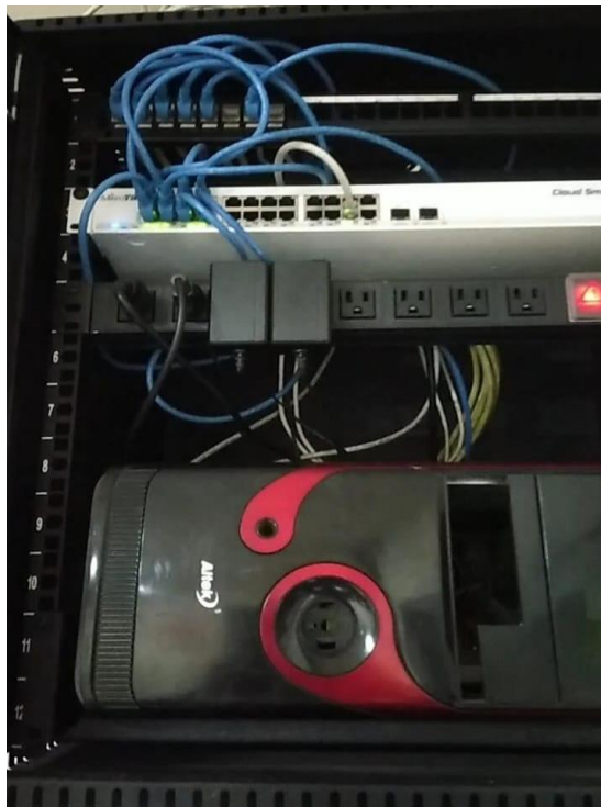
Figura 7.8 Rack y switch administrable.
