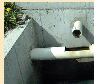
Figure 1. Low-flow/high-flow separation with over-shot pipe design. Low flows trickle from upper opening into horizontal pipe and are stored. High flows drop into concrete basin and are directed to Vegetative Treatment Area (VTA).
