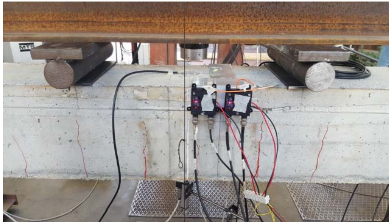
Fig. 7. Digital photo of the crack pattern at load cycle #06.
