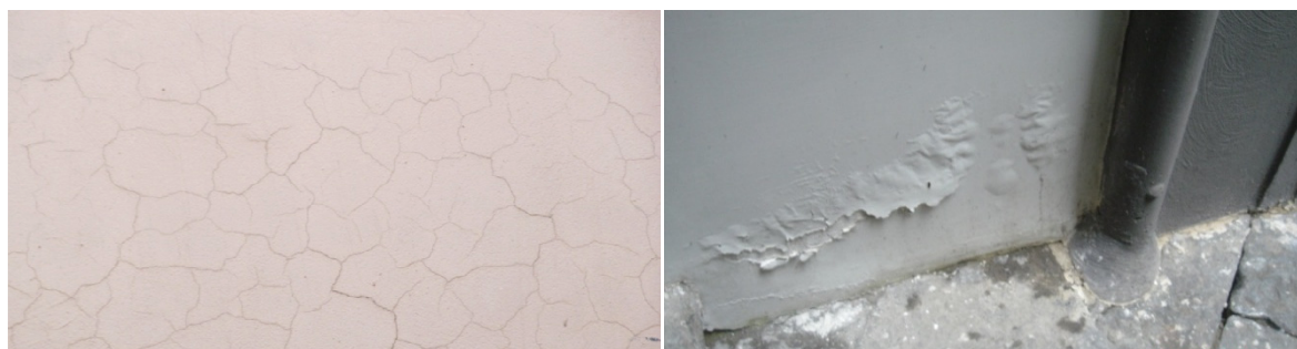
Figure 6-7: micro-cracks and rising dampness in a building with “Gs” solution
