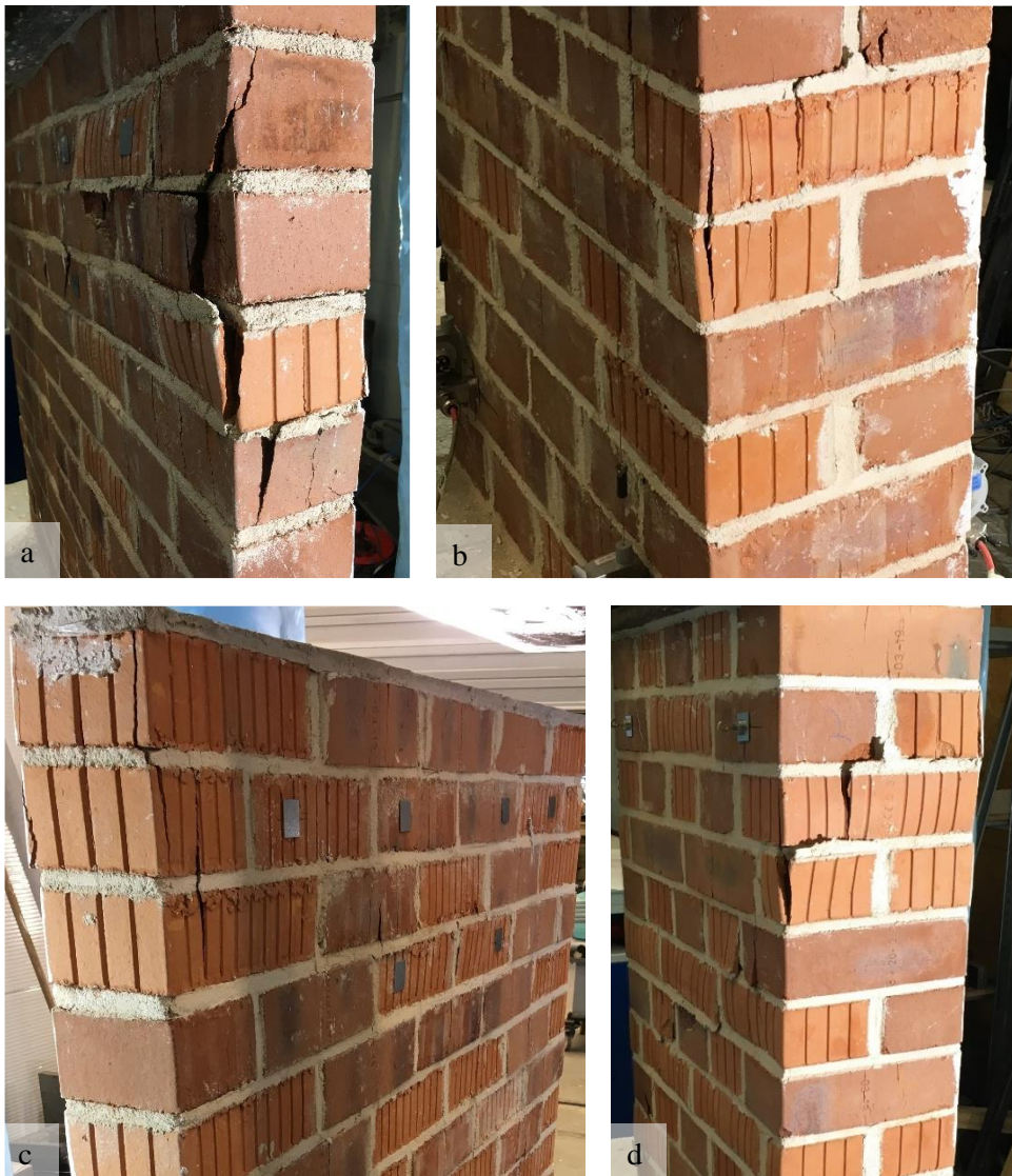
Fig. 4-17 Crack formation in the tests on walls with varying brick strength (a: sw-25-1, b: cb-25-1, c: sw-50-2, d: cb-50-1)
