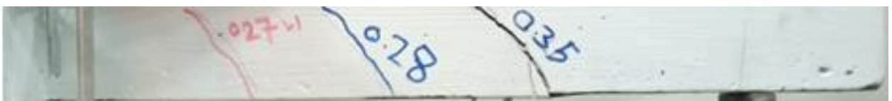
Figure 25. Crack pattern of spiral stirrups for spacing 60 mm
