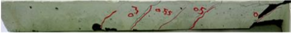
Figure 16. Crack pattern of closed stirrups for spacing 30 mm
