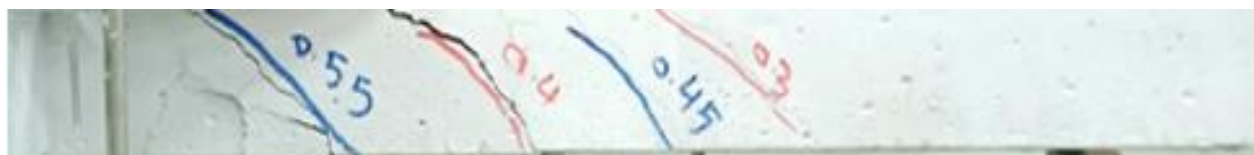
Figure 15. Crack pattern of closed stirrups for spacing 20 mm
