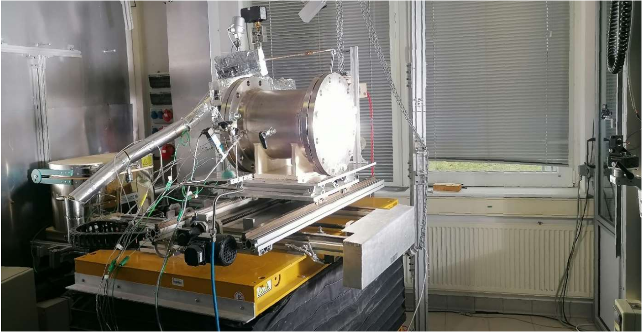
Figure 2: Solar heated solid oxide electrolyzer test platform in operation
