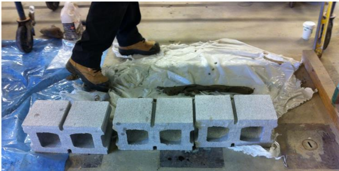
Figure A.3: The first course of masonry laid on a bed of mortar
