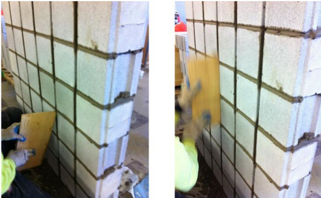
Figure A.5: Mortar being cleared from grooves using a piece of 3/8" plywood
