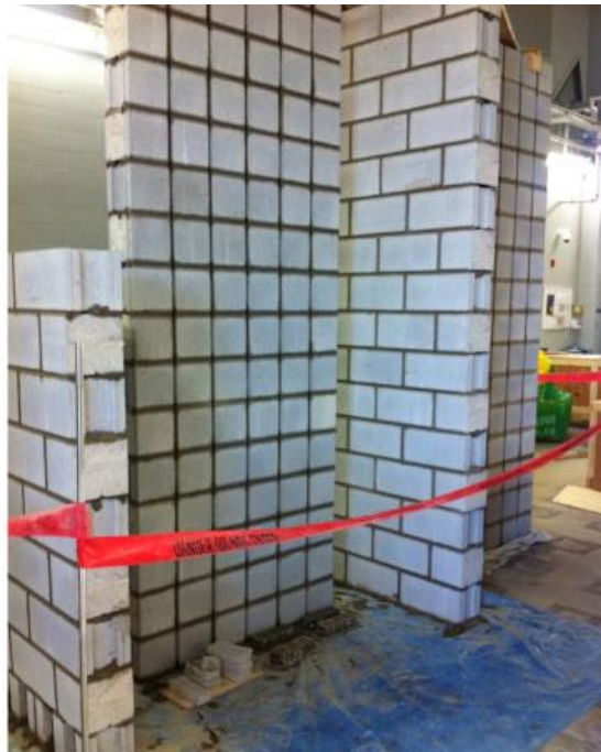
Figure A.8: Masonry walls at the end of the first day of construction
