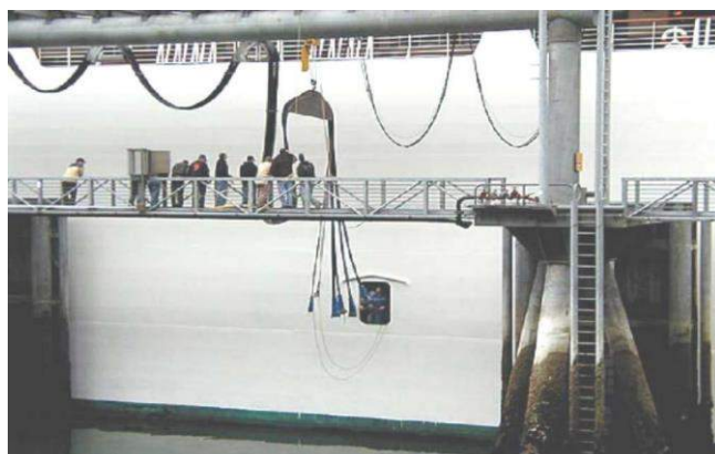
Fig. 3 Cold ironing arrangement in Juneau (Alaska)-2-
