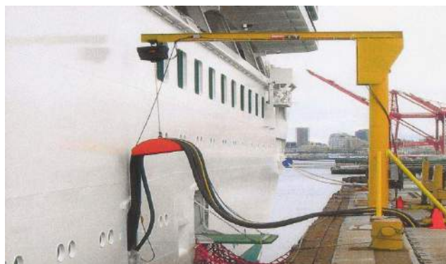
Fig. 1 Cold ironing arrangement in the port of Seattle (US)
