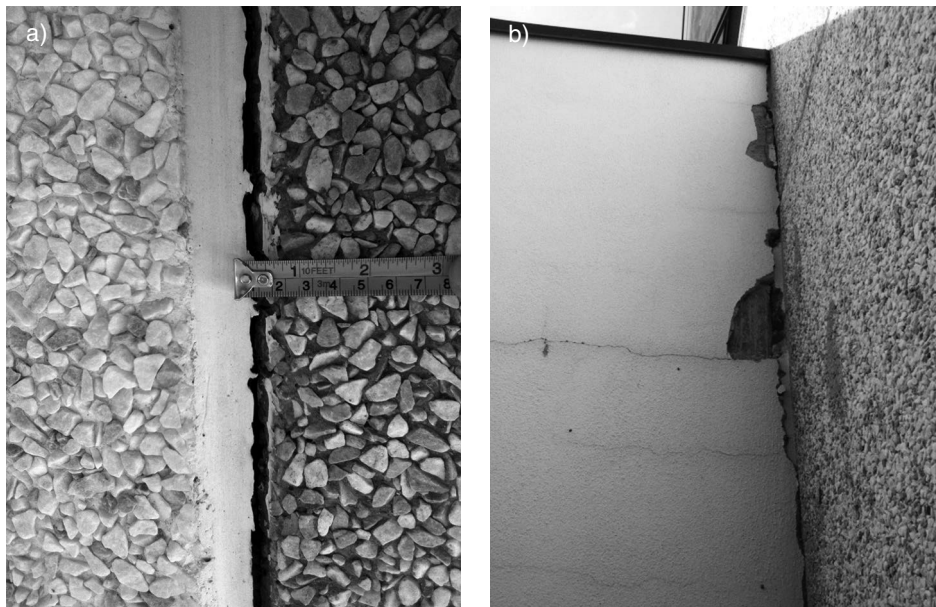
Fig. 32. Column-panel detachment (a) and vertical crack due to hammering effect among adjacent buildings (b). Distacco colonna-pannello (a) e fessurazione verticale dovuta a martellamento tra edifici adiacenti (b).
