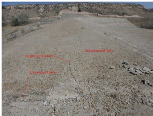
13. Transverse crack (foreground) in dam crest at STA 6+50 in foreground, looking left. Longitudinal crack extends from transverse crack about 20 feet to left. Top lift is unbonded left of transverse crack and downstream of longitudinal crack.
