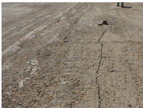
14. Longitudinal crack in dam crest near STA 8+50 and B-103, looking right from STA 8+60. This crack is about 0.25 to 0.5 inches wide and 25 feet long.
