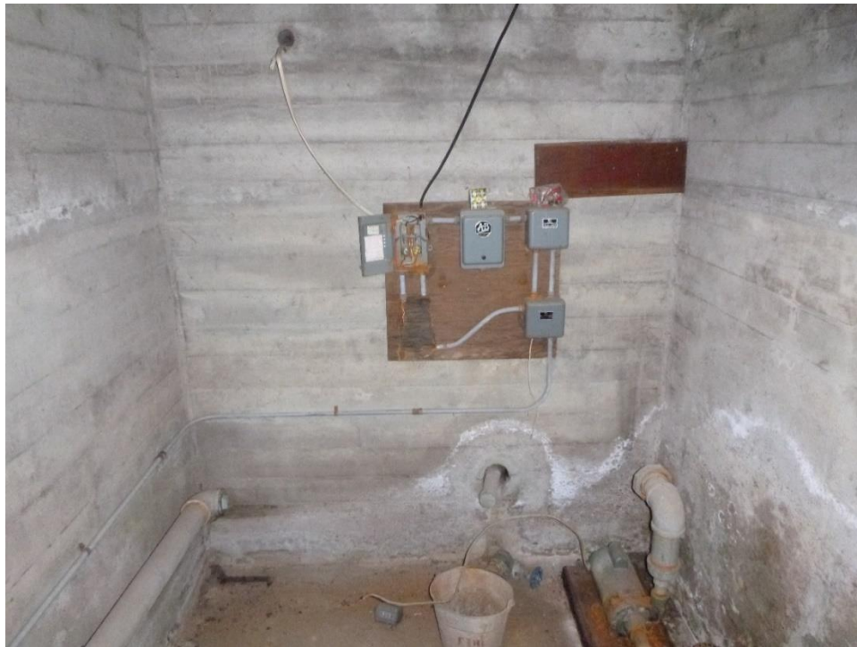
Figure 33. Interior of Old Well House (16-71) at base of the stairs, view from stairs.
