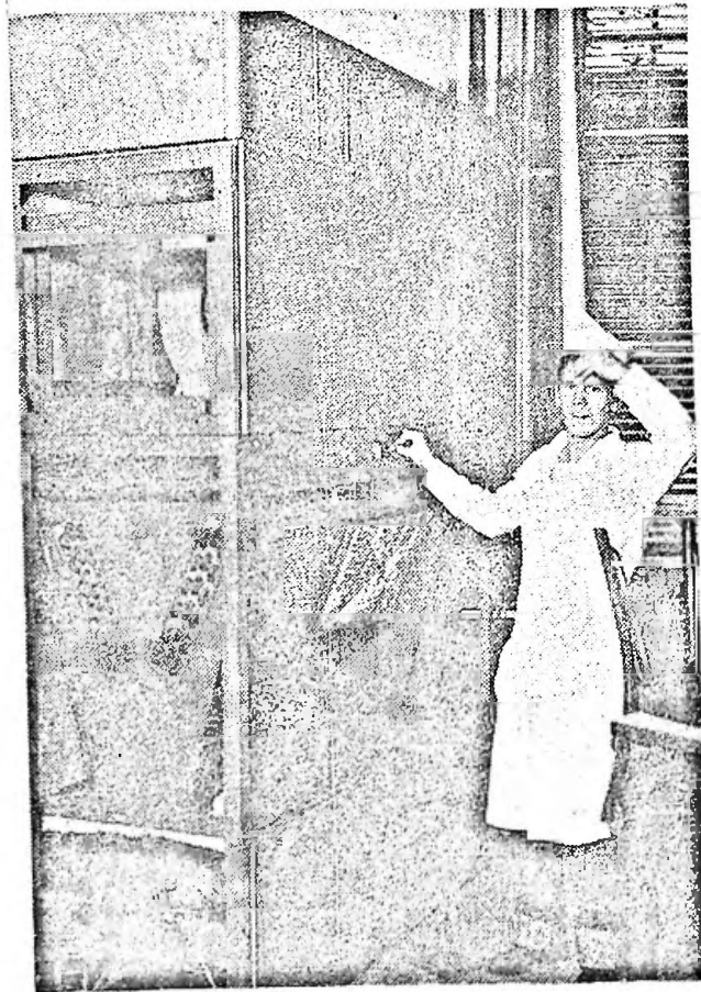
Bennie Mannon, busy boy at the Marshall College cafeteria, mops his brow and wishes this new air-conditioning unit in the main dining room were already in operation. However, the job isn't expected to be finished until the end of the month. The work is being done by Ferguson Brothers Plumbing and Heating Co. of Huntington.
