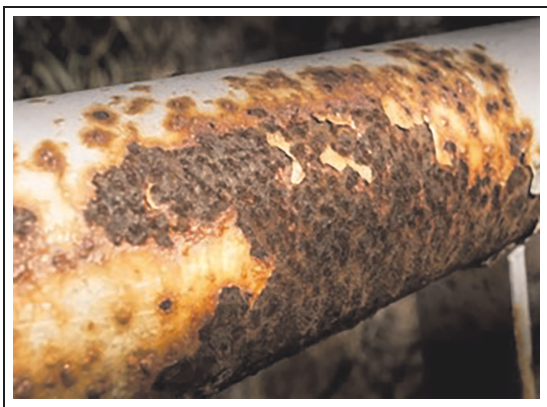
Figure 4. Corrosion in a pipeline and metal skin. 62
