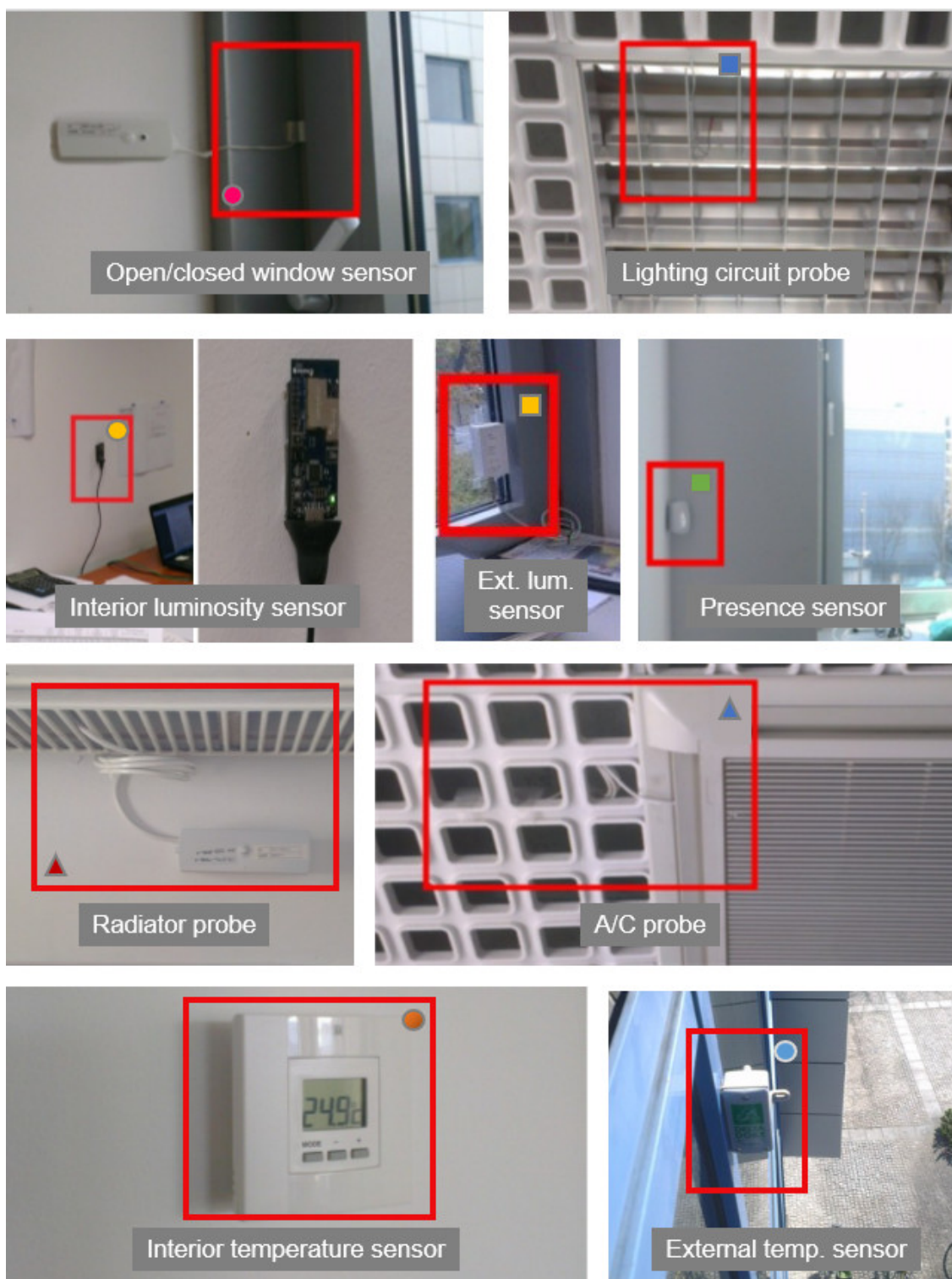
Figure 8. Pictures of several sensors used in the building in Warsaw.
