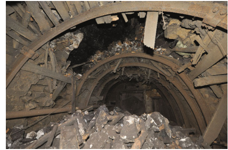
(b) Roof fall
