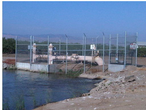
Figure 9. Pump station and valves to divert water from the reservoir into 3N or vice versa
