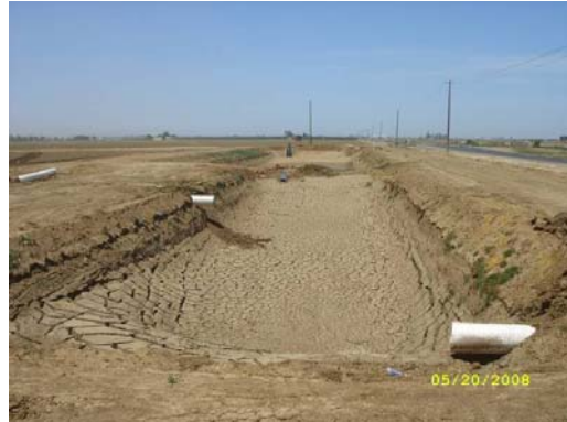
Figure 10. Westley Project tailwater collection and return system.
