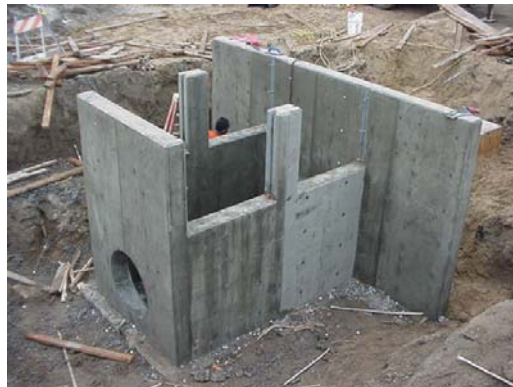
Figure 8. One flow control structure to the north of Fruit Avenue with weir length designed to pass high flows under system failure conditions.
