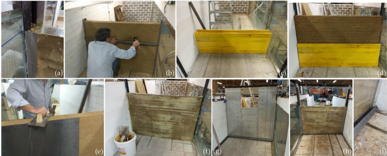
Figure 3. Images of the construction of the cohesive central core: (a) Placement of tape on the ‘vertical’ joints between the cohesive core and the metallic L profiles to avoid seepage; (b) Cut excess material from the core downstream face; (c) Formwork to compact the cohesive material; (d) Removal of the two upper panels of the formwork after compaction is finished; (e) Cut excess material from the core crest; (f) Protection of the downstream face and crest of the core with industrial vaseline (B-2 from Tecmasol); (g) Placement of downstream protection to simulate the downstream shoulder support; (h) Protection of the upstream face of the core with industrial vaseline (B-2 from Tecmasol); (i) Placement of tape on the horizontal joint between the cohesive core and the floor and placement of a metallic profile to avoid lifting and buoyancy of the tape.
