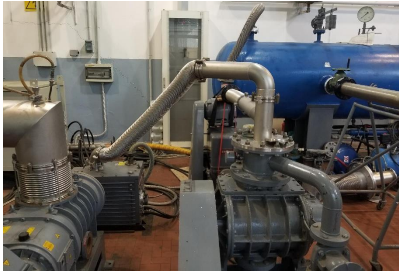
Figure 10 – Vacuum System: (a) Tank, (b) Rotary pumps.
