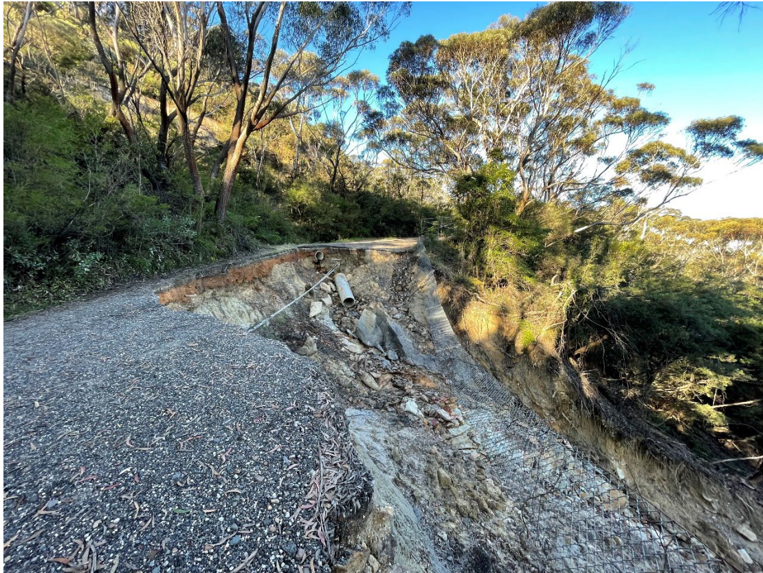
Figure 34. Slide on Glenraphael Drive, March 6. Photo by Larkin 8 th May 2022.
