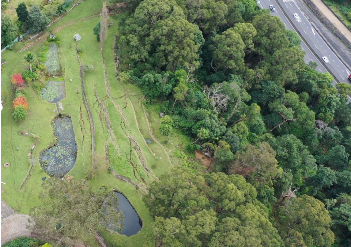
Figure 4. The three ponds area showing arcuate cracking on the 5 th May 2022 superimposed on landscaped terraces and retaining walls sculpted prior to 2011. The upper scarps of several debris flows can be seen along the tree line. RPA photo by Flentje.
