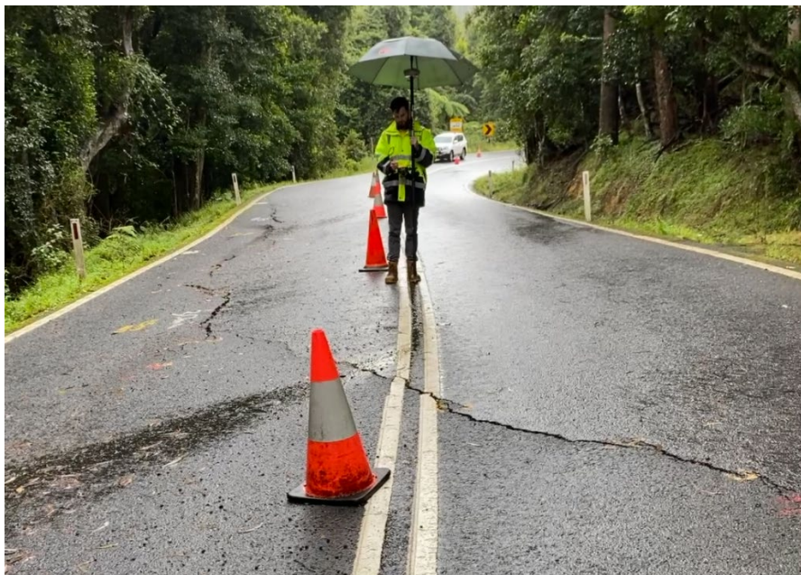
Figure 14. Macquarie Pass Trimble GNSS mapping of tension cracks and other relevant site features. Photo by Flentje, March 2022.
