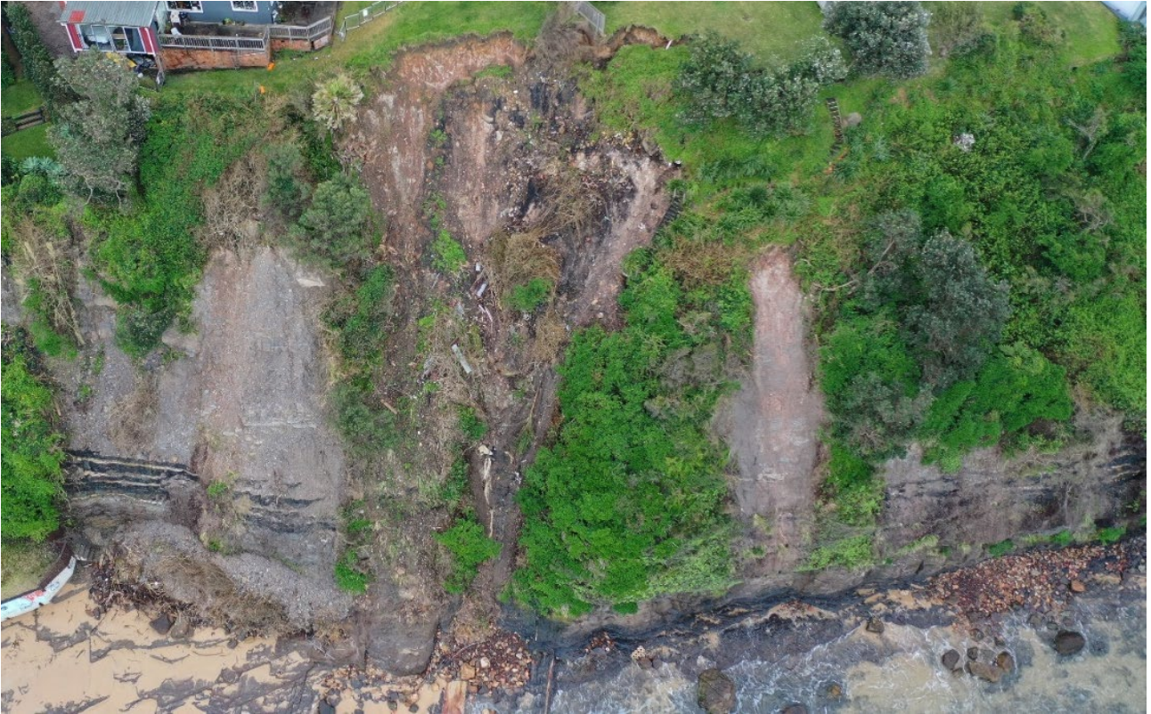
Figure 28. Fill and colluvial failure of coastal cliffs in the northern suburbs. In this section, the failure hazard is visibly apparent. RPA photo by Flentje 22 nd July 2022.
