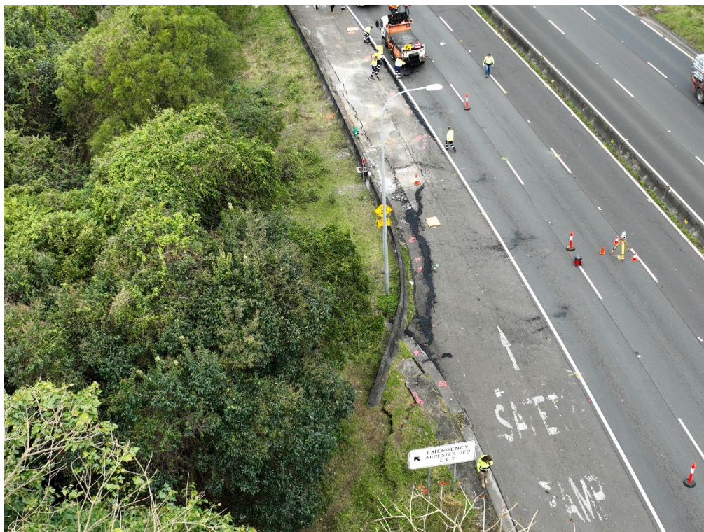
Figure 7. The southeastern quarter of the 810,000m 3 volume Site 141 landslide was reactivated between 1am to 3am on the 7 th of July 2022. Photo by Cox, 13/7/2022 at 11am during a southbound carriageway closure.
