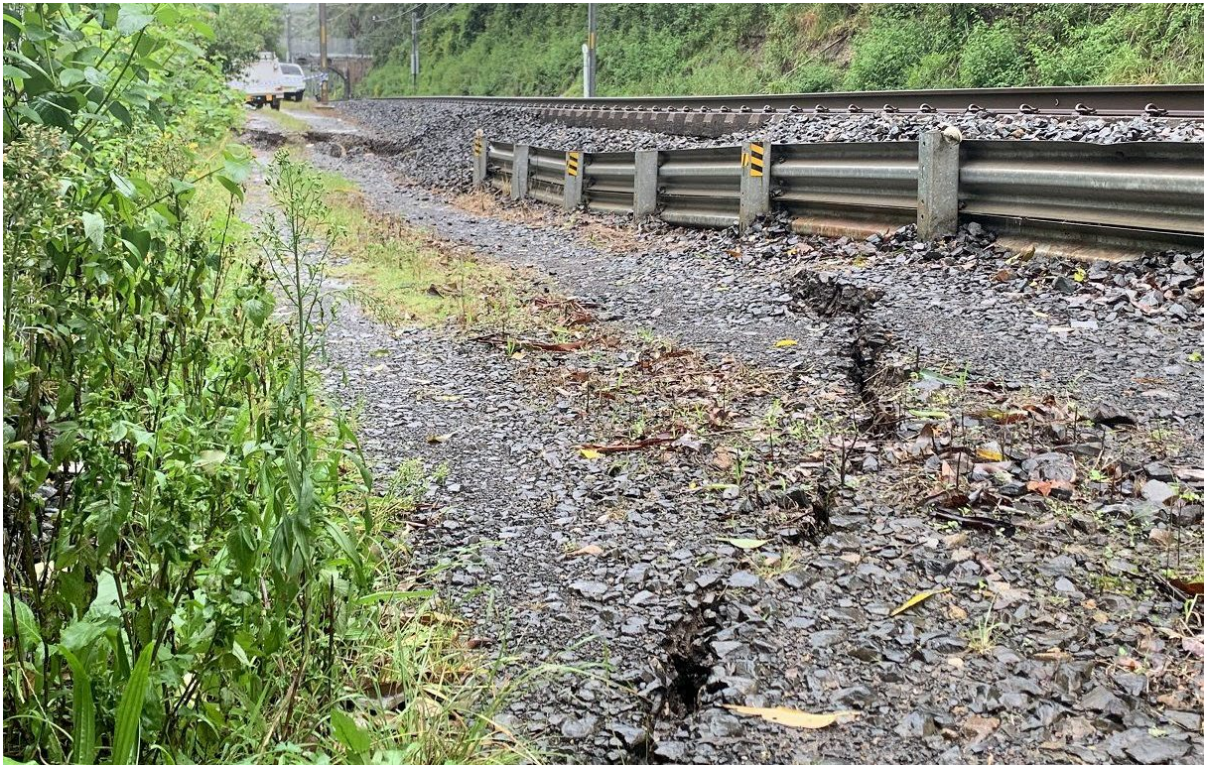
Figure 18. View towards Sydney (UP) at kilometerage 53.53km on the 7 th April 2022 at 3pm. Track, formation and Armco sag is clearly evident. Photo courtesy of S. Milling.
