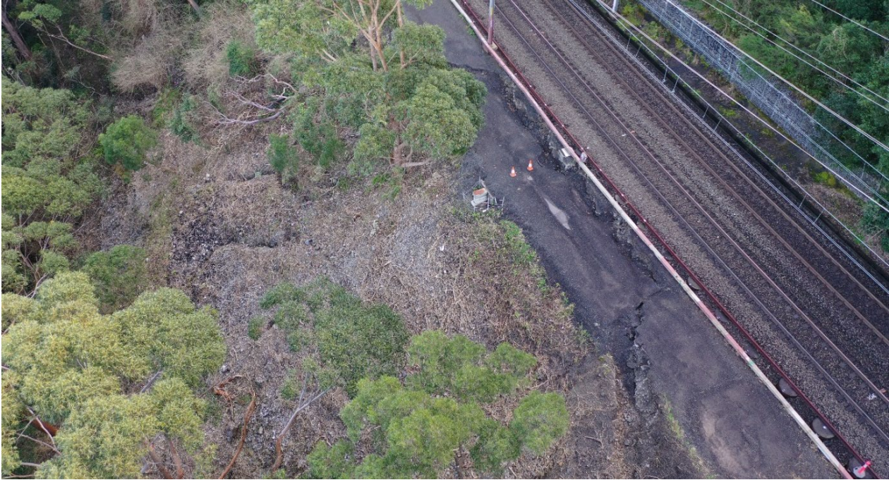
Figure 21. View to the west over the distorted upper slag embankment and headscarp of the Stanwell Park rail embankment failure at 56.300km. RPA photo by Flentje, 5 August 2022.
