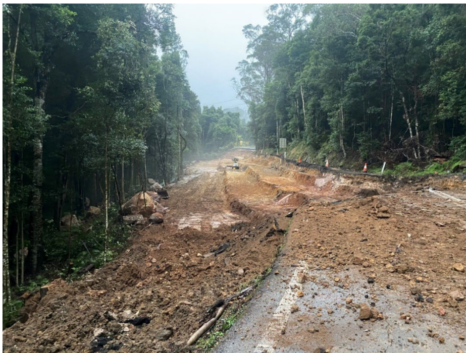
Figure 15. Benched excavation of landslide affected area at Macquarie Pass nearing completion. Photo by Boys, late April 2022.
