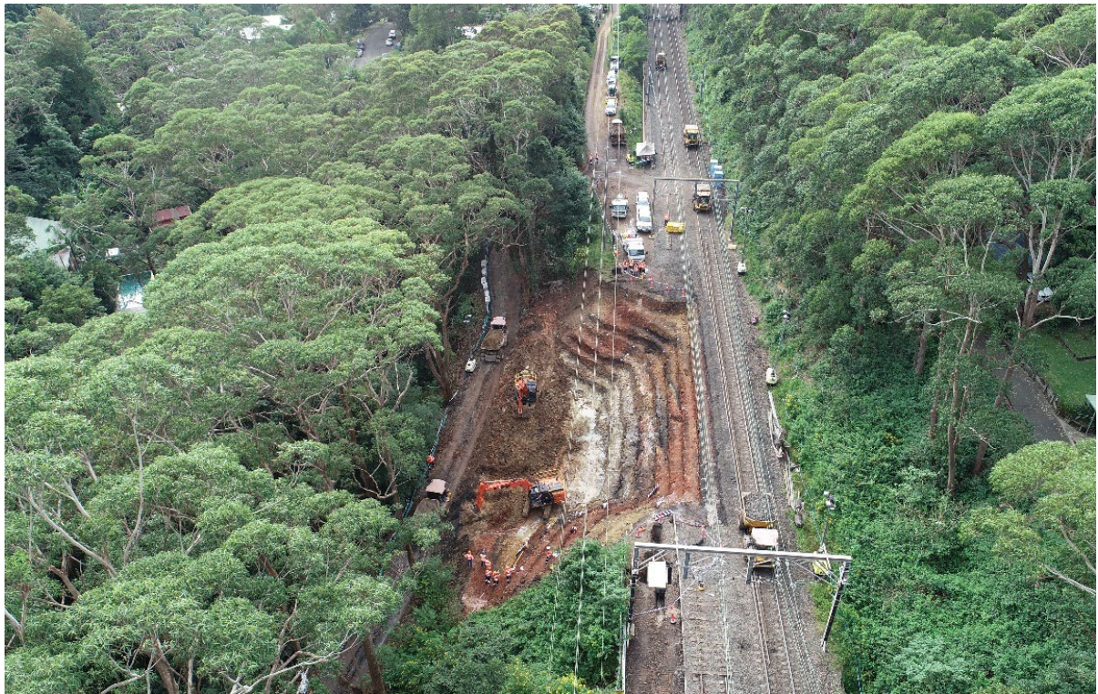
Figure 19. Looking towards Sydney above 53.7km on the 16 th April. The benched cut is near completion and lining with geofabric commenced in the same afternoon. RPA photo by Flentje.
