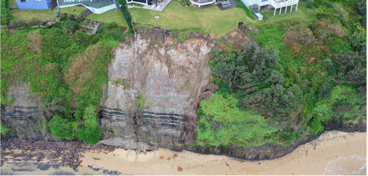
Figure 27. Fill and colluvial failure of coastal cliffs, northern suburbs. RPA photo by Flentje 22 nd July 2022.
