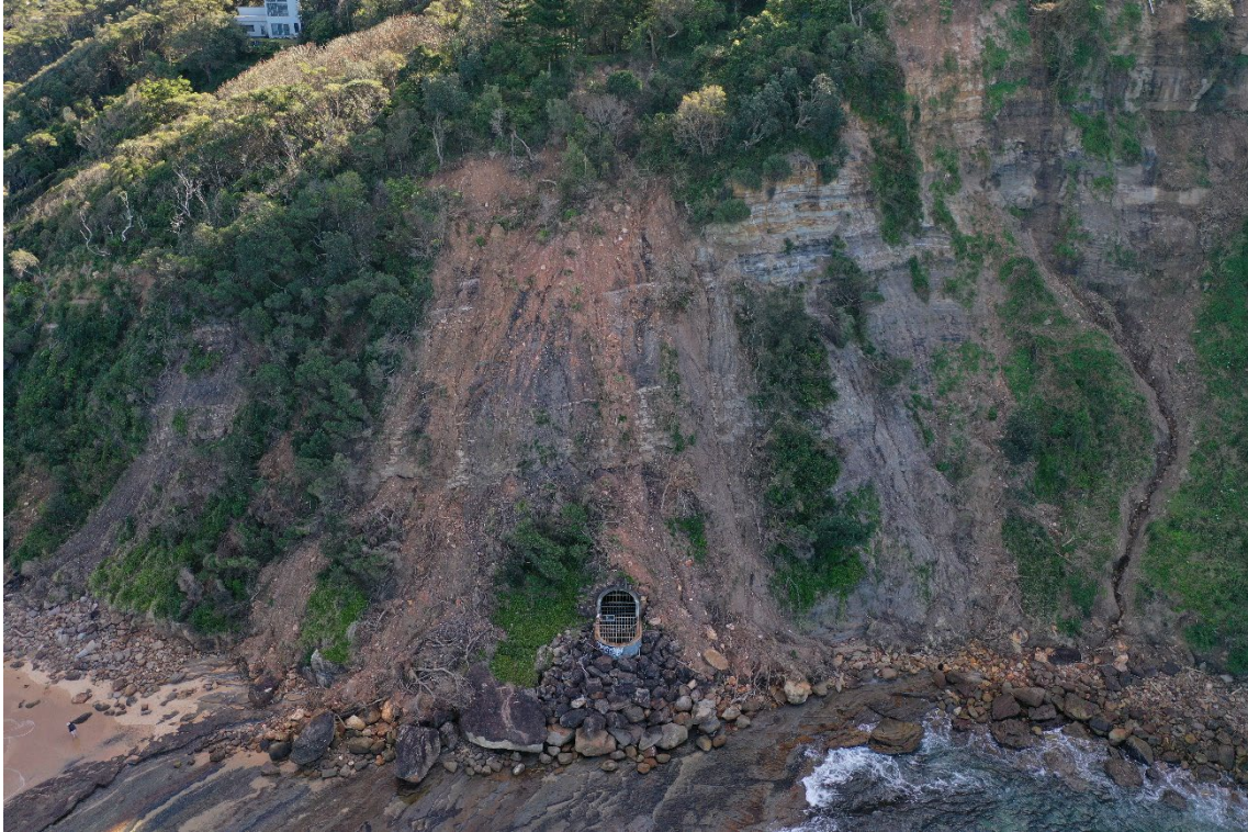
Figure 29. Failure of the colluvium mantle along the top of the coastal cliffs has resulted in debris flows and rockfalls onto the outlet of the Wombarra Drainage Tunnel, which is at the base of the cliffs in mid photo, at the north end of Wombarra Beach. RPA photo by Flentje 5 th August 2022.
