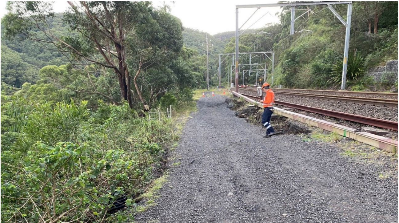
Figure 20. View southwest over the headscarp of the Stanwell Park rail embankment failure at 56.300km. Photo by Flentje, 14 April 2022.
