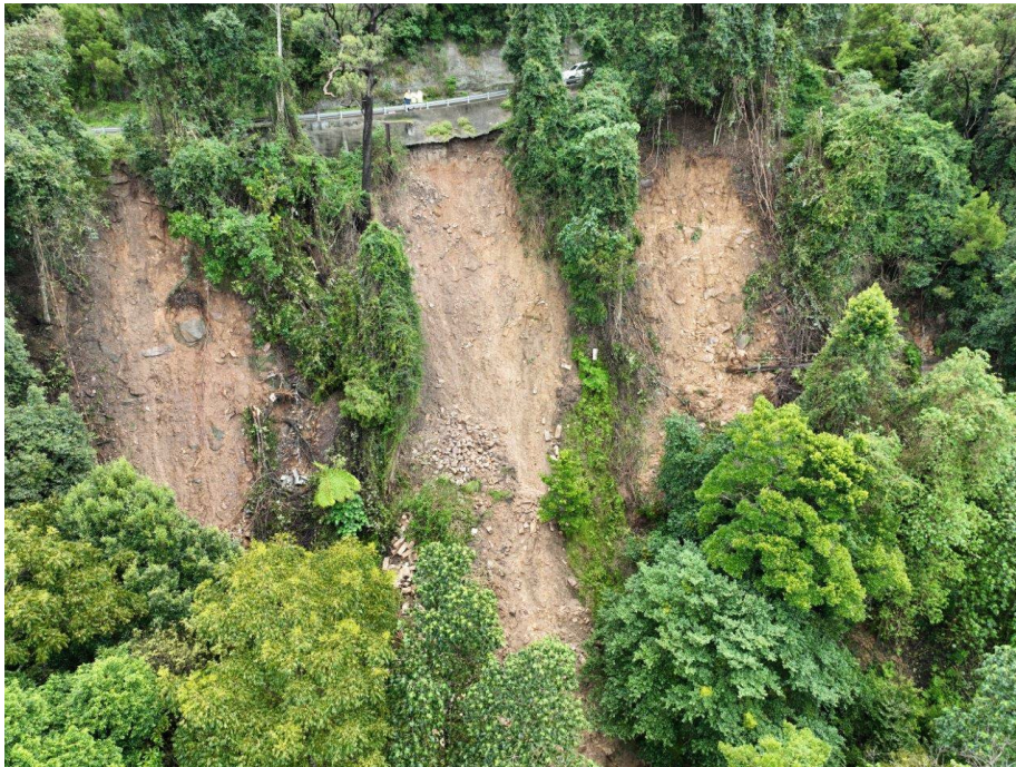
Figure 9. Very steep, approximately 75 degrees, downslope fill embankment slopes including the collapse of at least two old dry-stacked stone walls previously supporting Bulli Pass.
