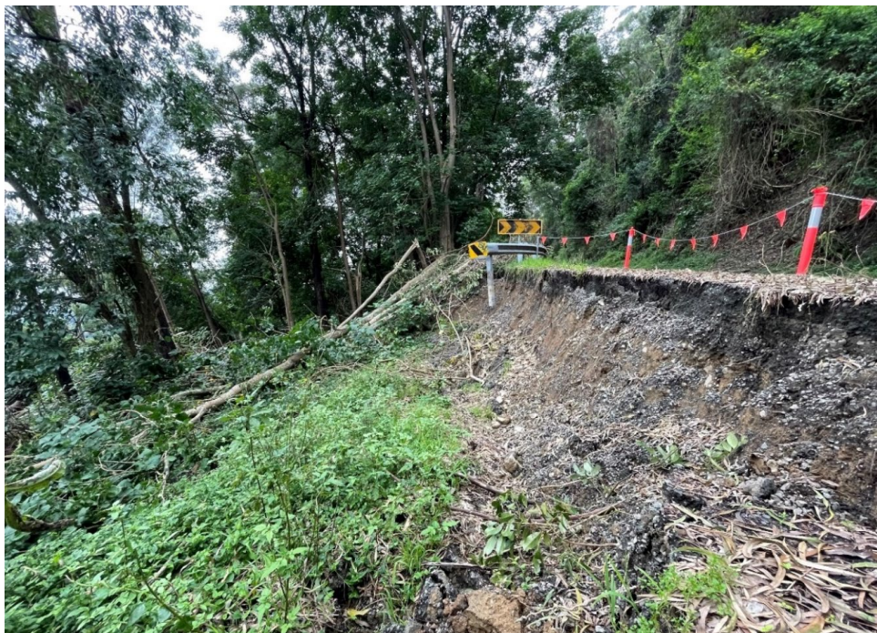
Figure 25. Major downslope slide on Harry Graham Drive. Photo by Larkin 30 th March 2022.
