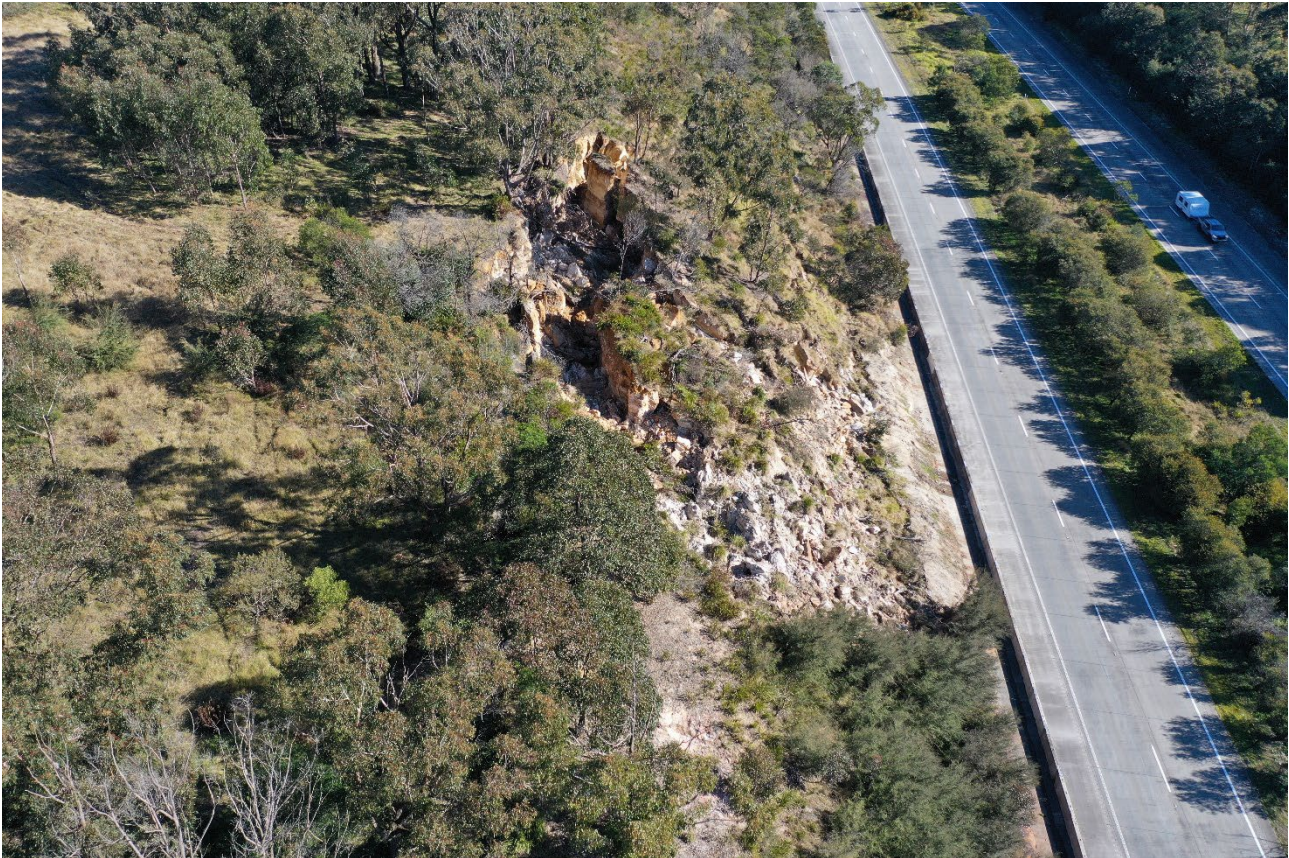
Figure 17. A Hawkesbury Sandstone cutting failure on the Hume Highway near Berrima. Initial inspections on the 7 th March were followed by geotechnical inspections on the 21 st March when the wider scope of the 10,000m 3 translational failure was acknowledged. Remediation has recently commenced. RPA photo by Flentje, 15 June 2022.
