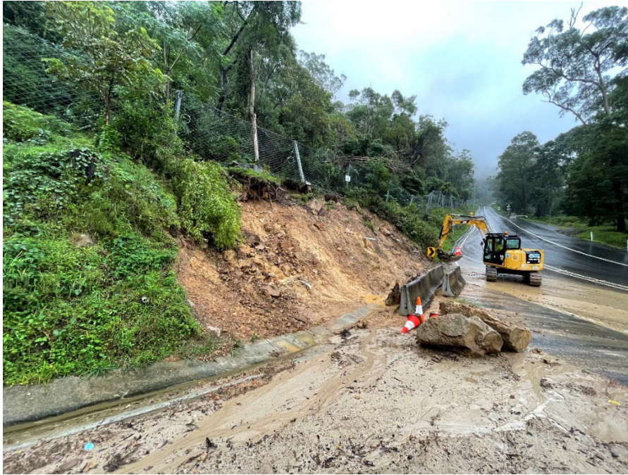
Figure 10. Bulli Pass failure on about day 4 of its activity, 5 th March during a day closure of the road.
