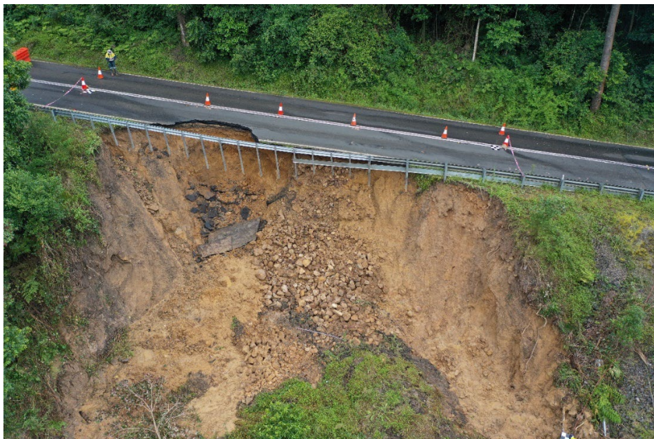
Figure 11. Barrengarry Mountain Road, close in view from a RPA aircraft showing the collapsed rockfill material, the unsupported Armco barrier and the flow like behaviour of the debris.
