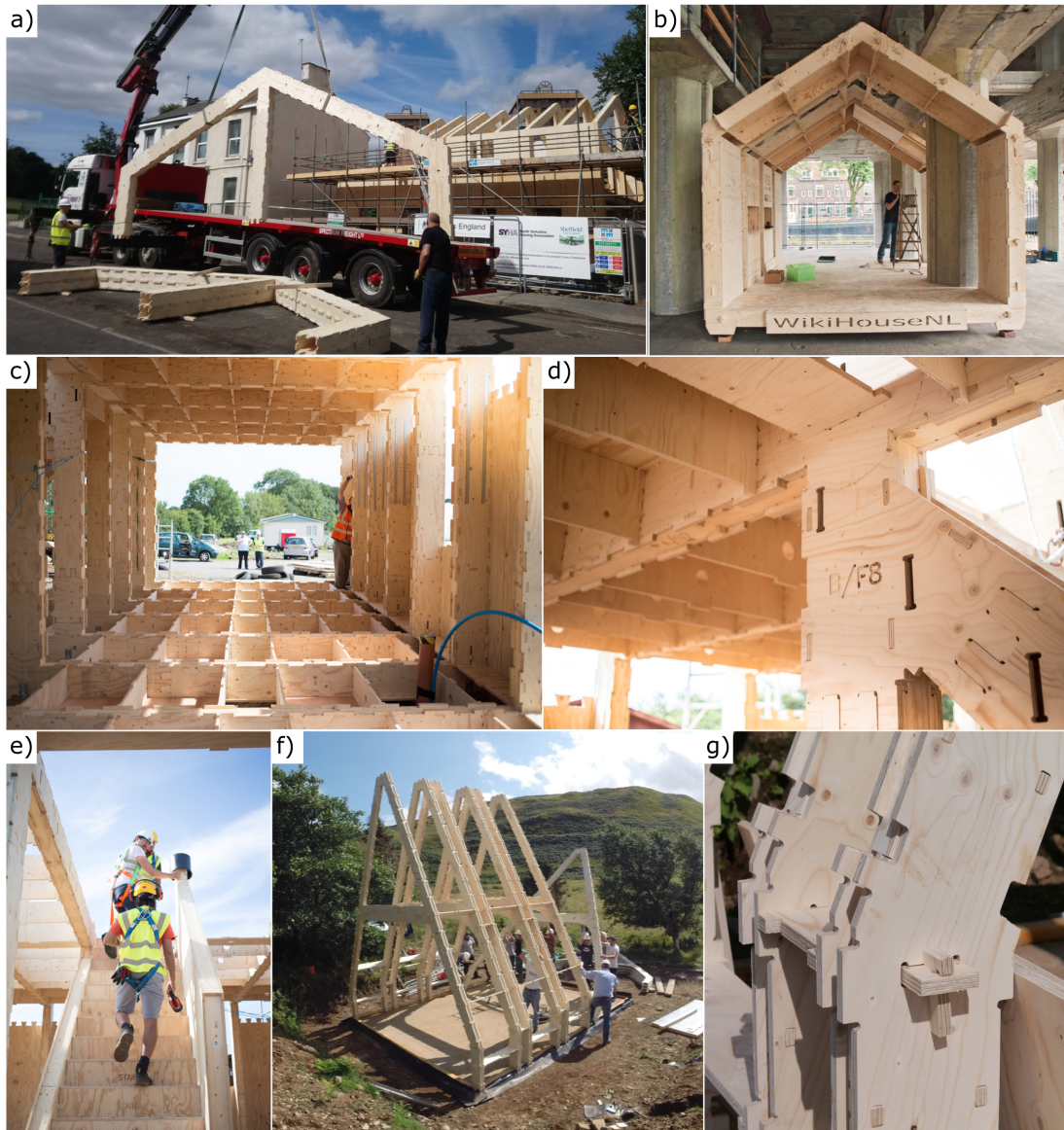
FIG. 1: Wikihouse buildings (courtesy of Open Systems Lab): a) South Yorkshire Housing Association, UK; b) Wikihouse Pavillon, Netherlands c), d) A-barn, Scotland; e), f), g) Farmhouse Warwickshire, UK. Further details at https://www.wikihouse.cc/Projects .
