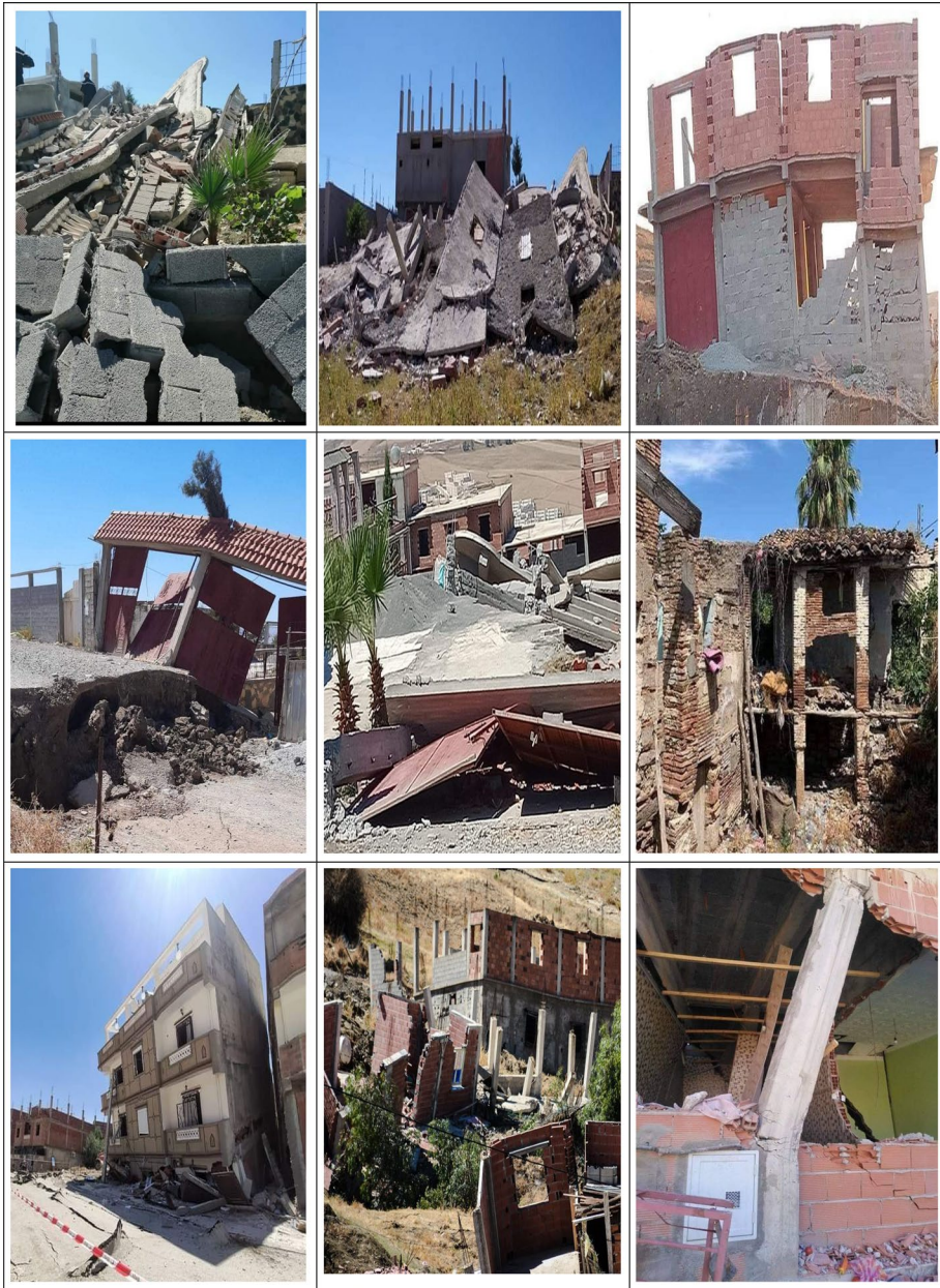
Fig. 1 Illustration of typical structure damage following the Mila earthquake
