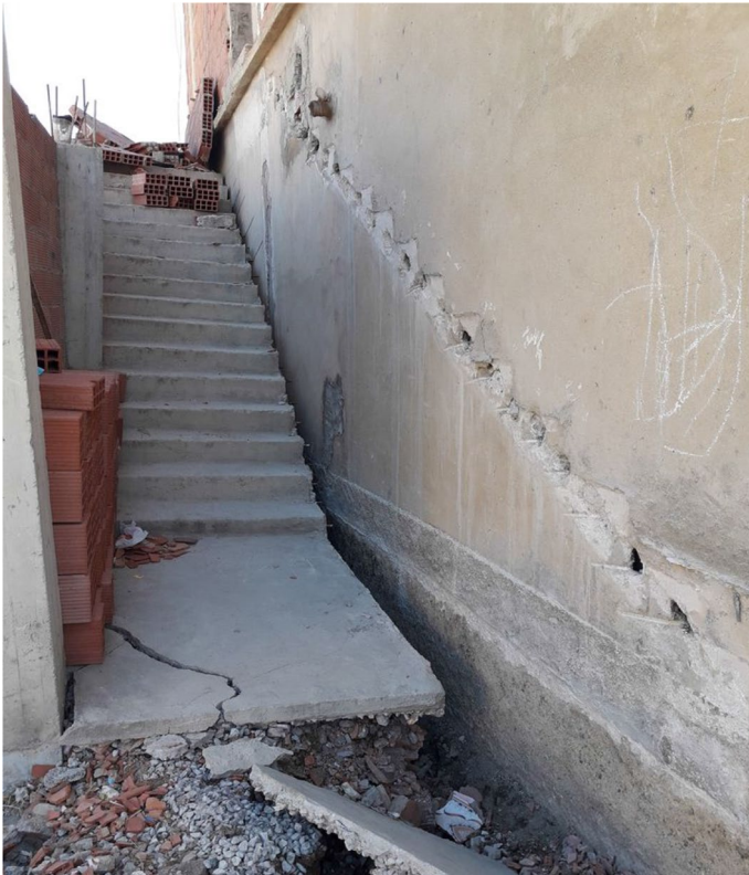
Fig. 18 Typical stairwell damage
