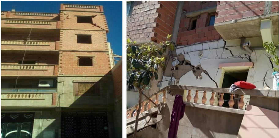
Fig. 15 Plan irregularities caused damage to the connecting components
