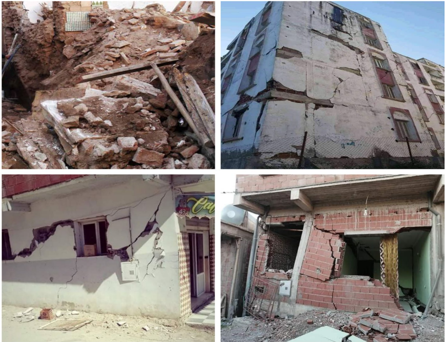
Fig. 14 In-plane and out-of plane damage
