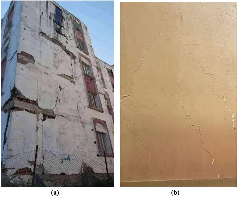
Fig. 22 Exterior a and internal b cracks on the eastern stairwell
