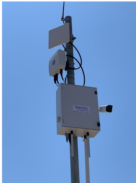
Figure 2.1: RSU with a camera installed and its components
