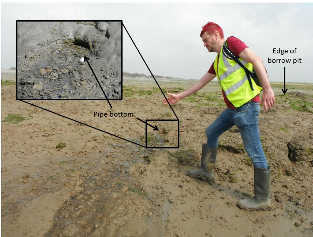
Figure 7.7: Water flowing from the bottom of a pipe (insert) through the bank of the borrow pit (looking north-eastwards) in June 2014 (photograph: H. Burgess).
