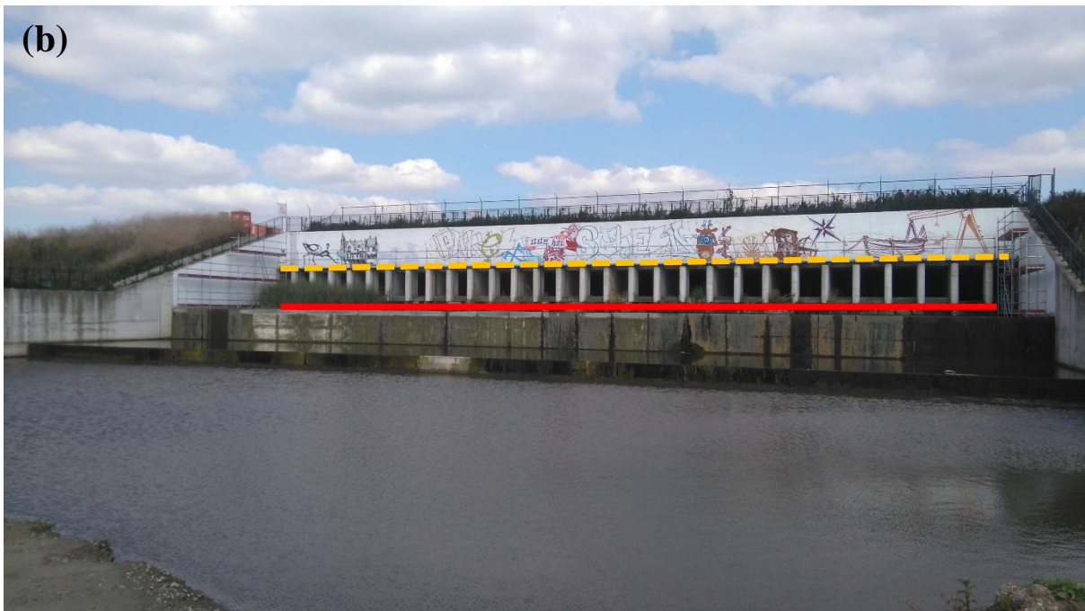
Figure 2.1: (a) The estuarine side, looking upstream, and (b) the landwards side, looking towards the estuary, of the sluices for a controlled reduced tide scheme to be implemented on the Scheldt estuary, Belgium as part of the Sigma Plan. Note the large difference in elevation between the two sides of the sluice. The water level in (a) is approximately level with the bottom of the white pillars in (b), marked by the solid red line, and the top of the sluices is marked on both by the yellow dashed line which is approximately 20 m long (photograph: J. Dale).
