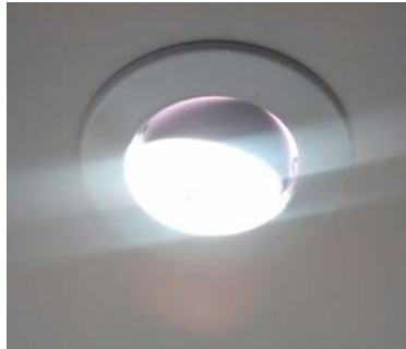
Figure 65: LED pot light at AS.C01's basement living space
