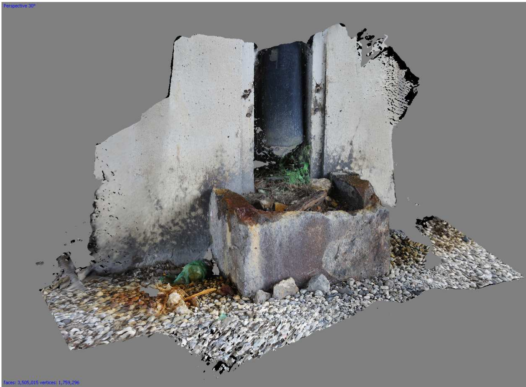
FIGURE 4.2: Raw photogrammetry scan of another highway detail
