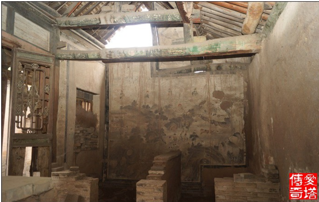
Figure 9 The fresco on the wall in the main hall of Zhenwu temple. Because of leakage, the fresco is covered by mud, source: http://blog.sina.com.cn/s/blog_4a877d4d0102ew9h.html
