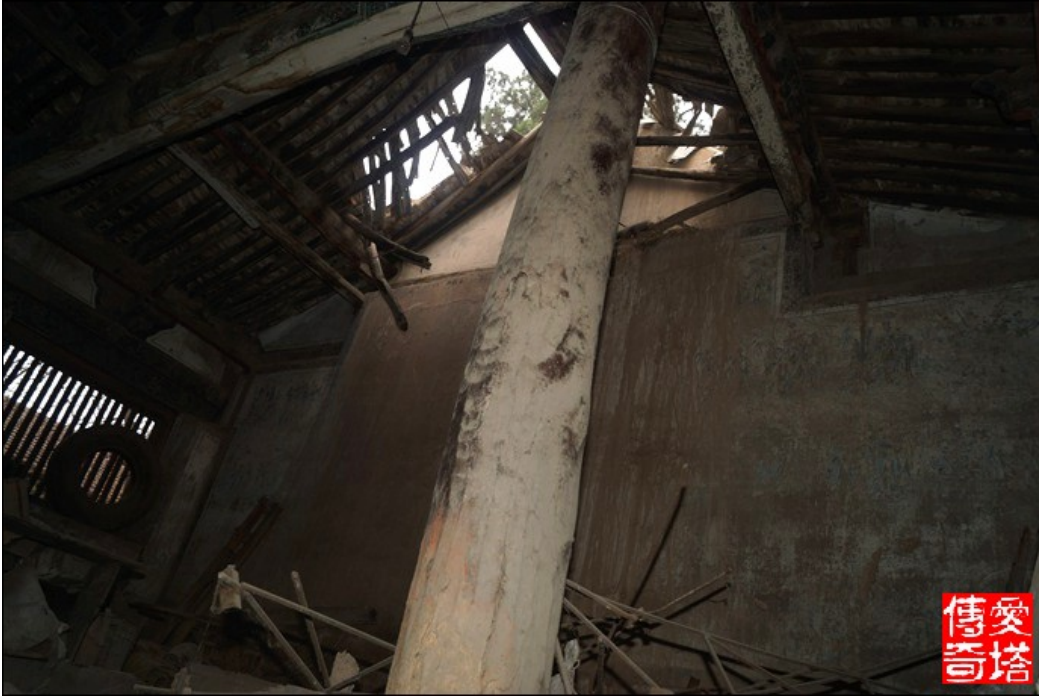
Figure 7 The collapse on the roof in Miaoju temple, source: http://blog.sina.com.cn/s/blog_4a877d4d0102ew9h.html
