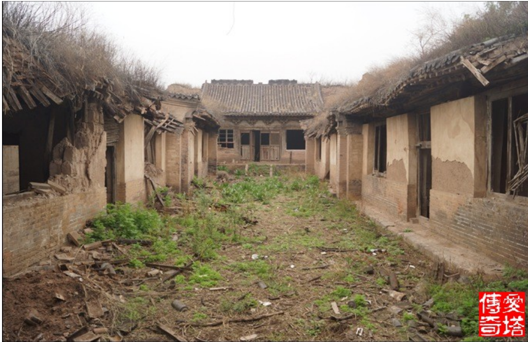
Figure 8 The back hall and side halls of Zhenwu temple. Buildings are dilapidated, and the entire courtyard is full of tiles and wooden component that have fallen down, source: http://blog.sina.com.cn/s/blog_4a877d4d0102ew9h.html
