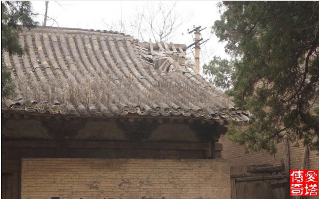
Figure 4 The collapse on the roof of the main hall of Miaojue temple, source: http://blog.sina.com.cn/s/blog_4a877d4d0102ew9h.html
