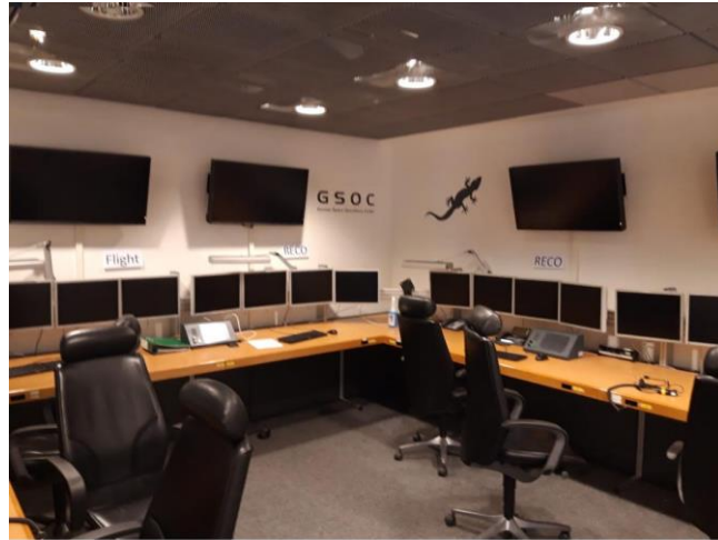
Control room at DLR
