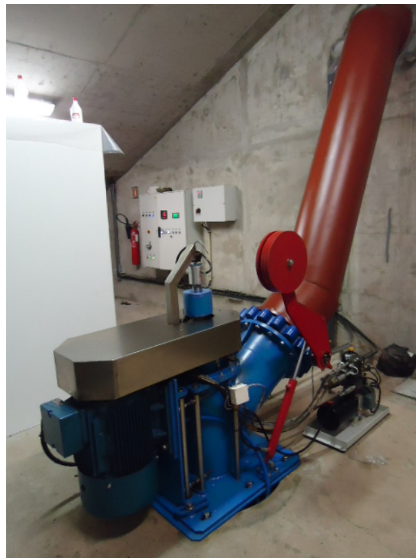
Figure 3.3: 15 kW hydroelectric generator in the CCVB.
