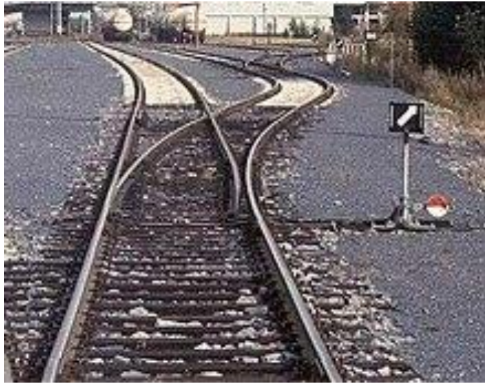
Fig. 1.1 Railway switch in an operational railway environment
