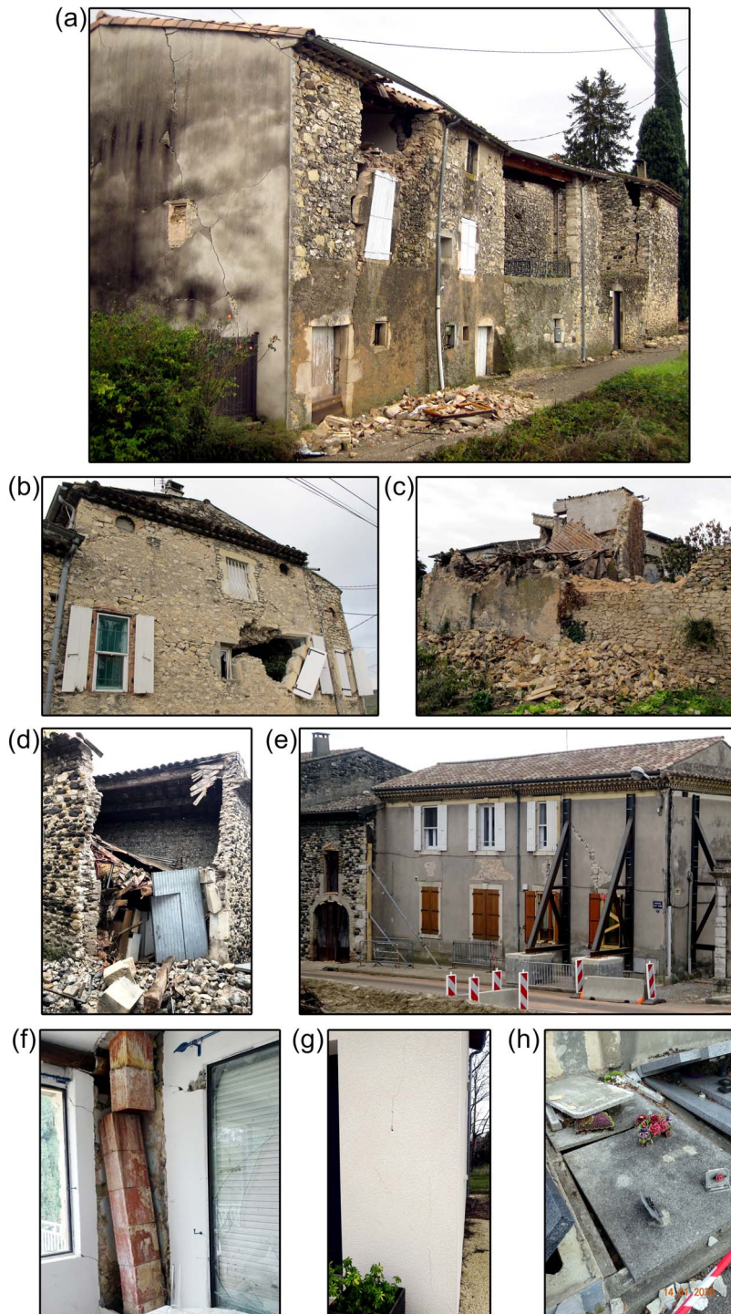
Figure 8. Types of damage observed in the zone of maximum intensity VIII, locality of Le Teil, from La Rouvière district (photographs a, b, c) to the Mélas district (photographs d and e), and on the road connecting the two districts (photographs f, g, h).
