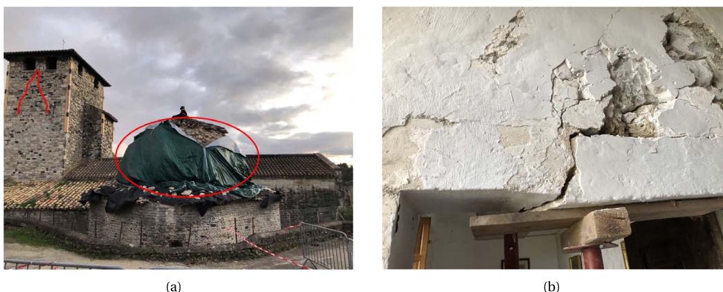
Figure 8. (a) Saint-Etienne of Melas church (assumed construction date: 11th century): degradation of the cover of the baptistery in the red ellipsoid, cracks in the bell tower indicated by the red lines. (b) Castel of Saint-Tomé (assumed construction date: 14th century), broken lintel.
