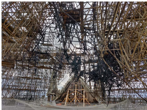
Figure 11. Steel scaffolding (surrounding the spire before the fire) deformed by the high temperatures (photo by Damien Deldicque and Jean-Noël Rouzaud).
