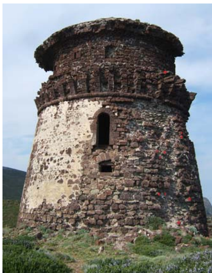
Fig. 4. In the conical base, left side of the image, remains of the covering plaster still with good adhesion of the masonry, are visible; on the right side it is evident the zone where a portion of the external wall fell, uncovering the wall core structure. With red asterisks are marked the stone blocks that in 2010 were still on site and that in the 2013 survey fell down.
