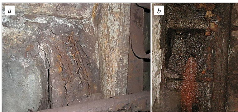
Fig.4. Corrosion of tunnel lining made of reinforced concrete (a) and cast iron (b) (photo by E. Yu.Shatskaya)
