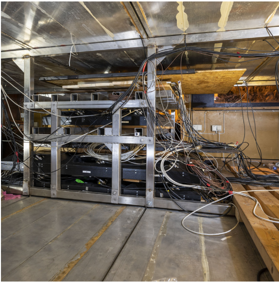
Fig. 1. Photo of the central part of the current NEMESIS setup.
