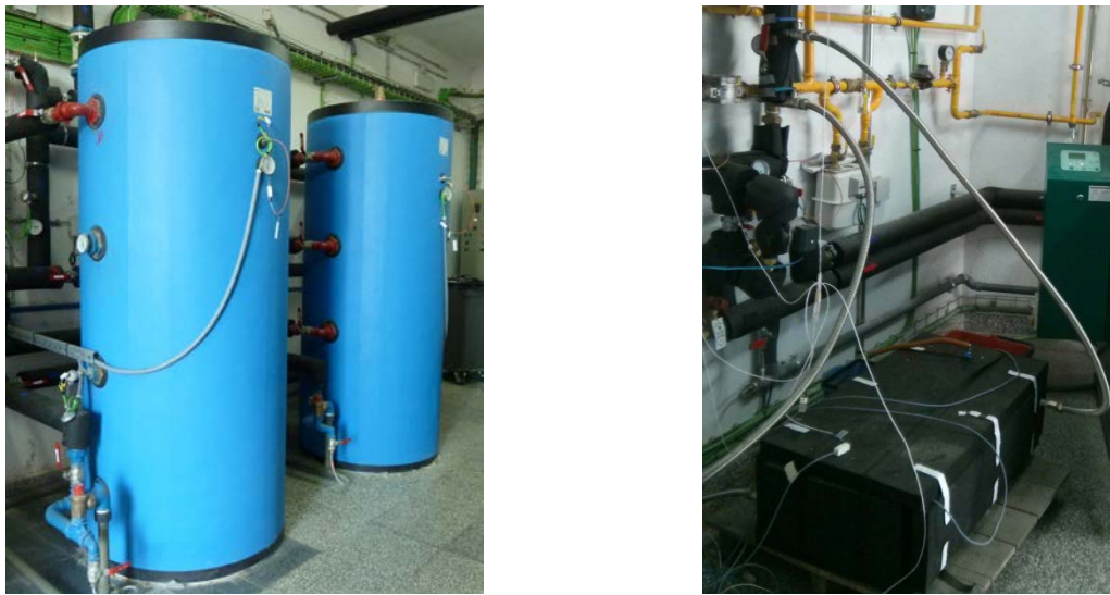
Figure A.6 – Thermal Storage Module: hot water tanks (left) and LHTES (right).
