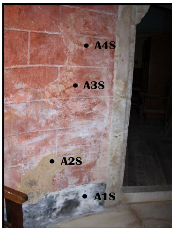
Figure 10.7: Area characterized by efflorescence salts and degradation of the plaster. Four mortar samples were selected to be analyzed by Ion Chromatography after performing the soluble salt tests.
