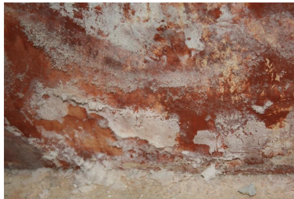
Figure 3.13: Extensive efflorescence salts observed in the secondary vault of the church.
