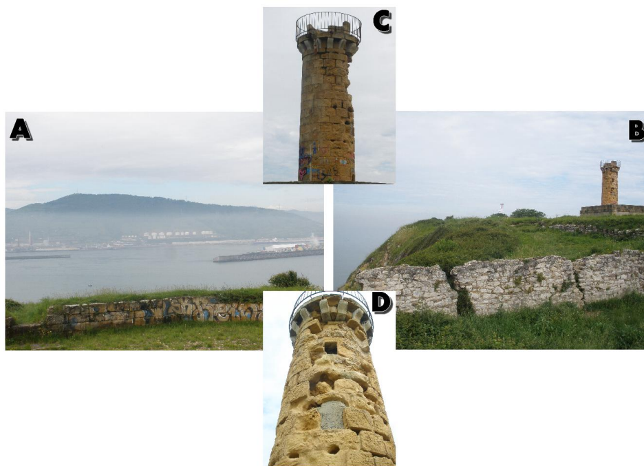
Figure 7. Location and views from La Galea Fortress, showing A) and B) the direct influence of the marine aerosol, surrounded industry and ships traffic C) and D) evidences of the poor conservation state of La Galea Fortress tower.
