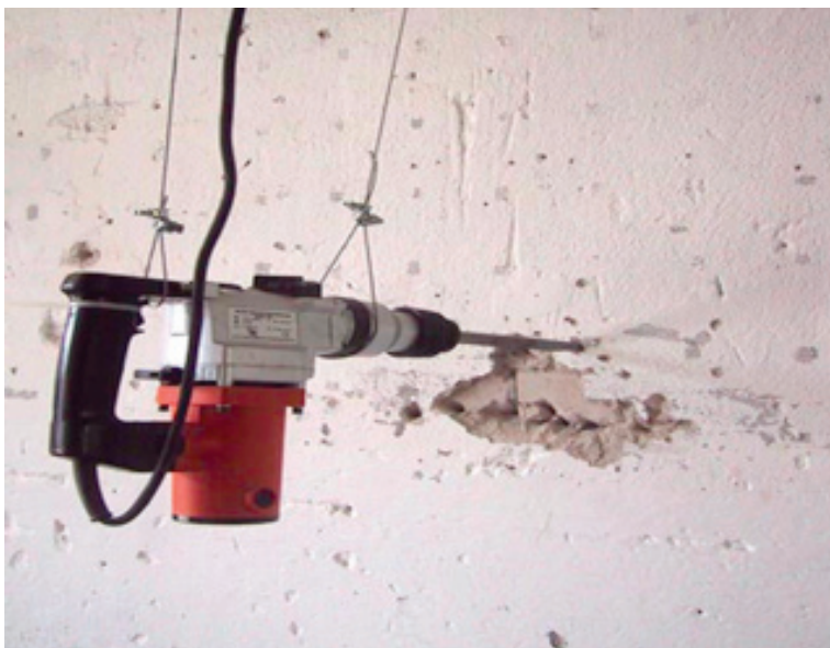
FIGURE 3: In Jonah Brucker-Cohen's Alerting Infrastructure! visits to the website of a gallery space actuate a large pneumatic jackhammer that "deconstructs" the physical building that the website represents.
